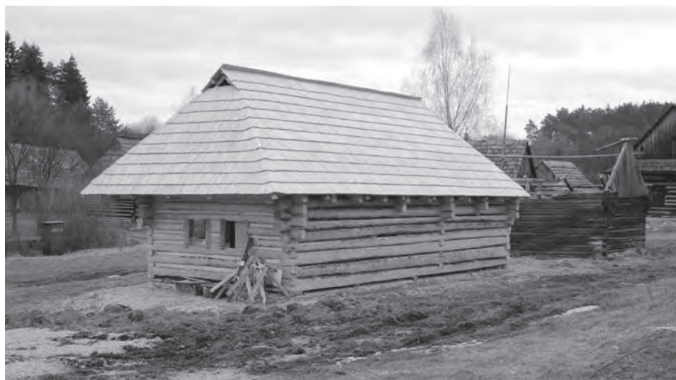
Obr. 7. Objekt z Trebostova v Múzeu slovenskej dediny počas stavebných prác. Foto J. Neplech, 2013 Pic. 7. Building from Trebostovo in the Museum of the Slovak Village during building work. Photo J. Neplech, 2013
